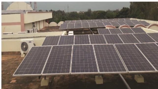
Fig. 3. On-grid solar power plant at Karunya Institute of Technology and Sciences -Part A
