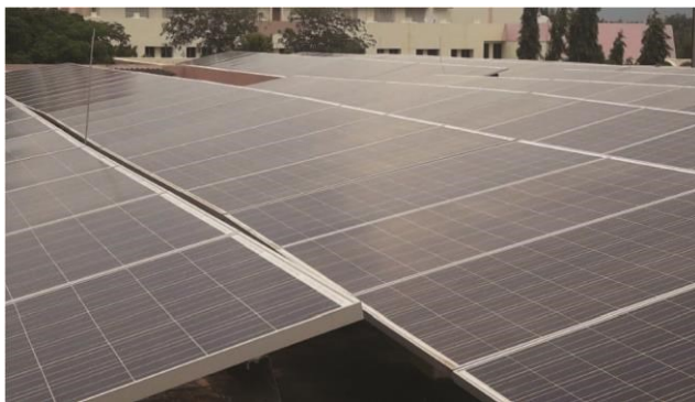
Fig. 4. On-grid solar power plant at Karunya Institute of Technology and Sciences-Part B.
