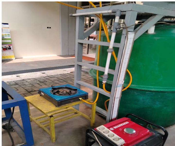
Waste processing equipment into gas, Faculty of Engineering, Pancasila University
