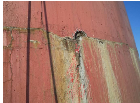
Figure 3b. Chimney wall destruction
