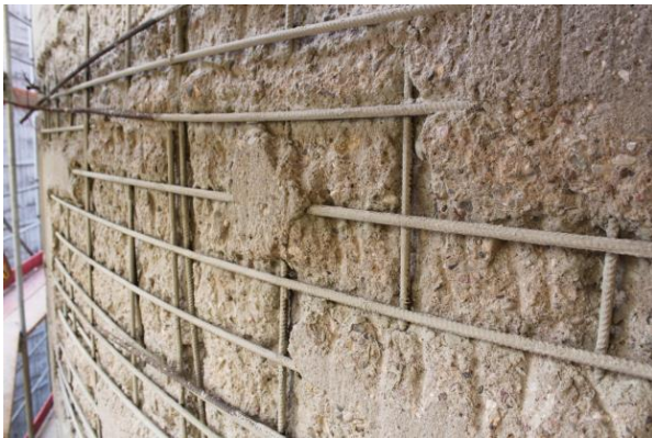
Figure 3a. Concrete cover and corroded steel bars of silo wall
