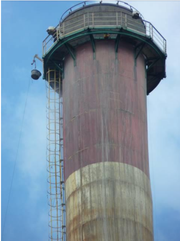
Figure 4a. Chimney before repair
